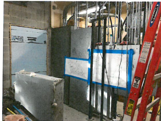
Increased Capacity In Electrical Room
